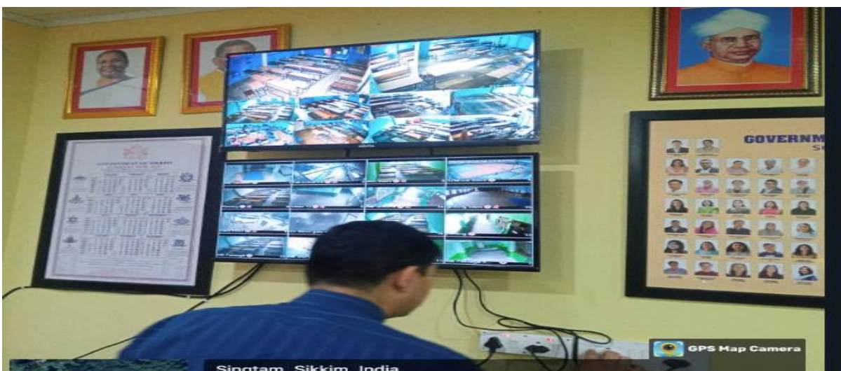
10 CCTV cameras with SITC 32 inch screen installed at 24 PM Shri Schools:
